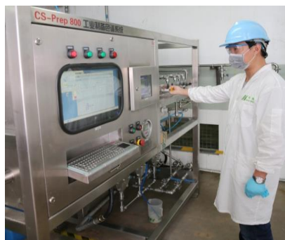
Advanced Process Control System
